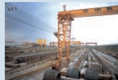
Phase 1 of the Western Delta Route (Under construction) 珠江三角洲西岸幹道第一期 (建設中)
